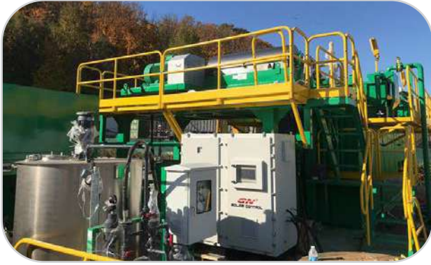
US 15 m 3 Slurry Treating System
