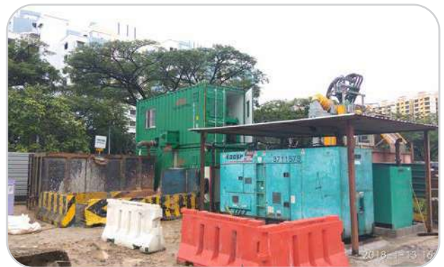
Singapore 5 m 3 Slurry Treating System
